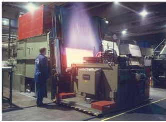
Box / Sealed Quench Furnace Installation
